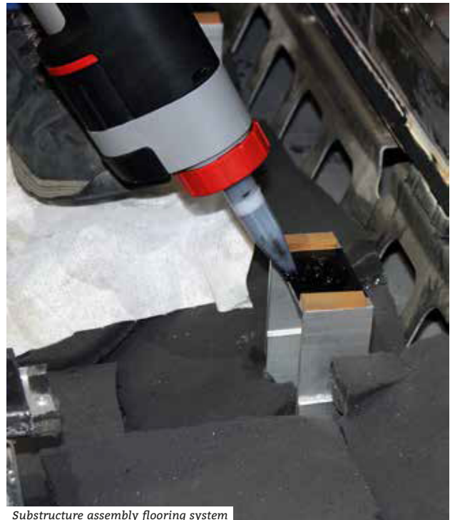
Substructure assembly flooring system
